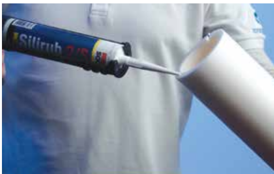
4.3 Carefully apply sealant/adhesive to the longitudinal joint, and the end of the second insulation tube, preparing the butt joint to the next item of insulation. In this example the 50mm / 2" tube.
