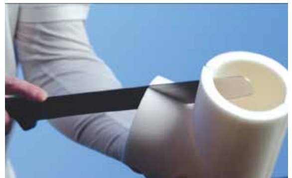
2.4 After the sealant has cured, the fitting is cut across the internal throat of the elbow, and then installed around the pipework elbow.
